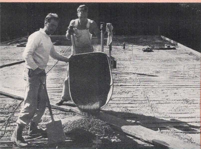
A drawback of panel heating is that alterations in the system, if needed, are difficult and costly, making correctness of original design doubly important.
