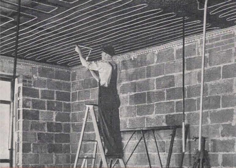
An efficient radiant panel heating system must not only be carefully designed, but should be installed exactly in accordance with the calculations.
